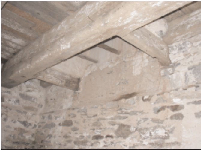
Photo 4. Framing of the hood of the jambless fireplace in the spring house.
