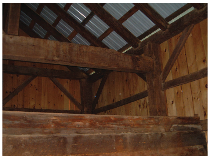
Photo 2. Fort barn interior; view showing corner post w/ ETJ and adjacent dropped tie beam bent (author 2012).
