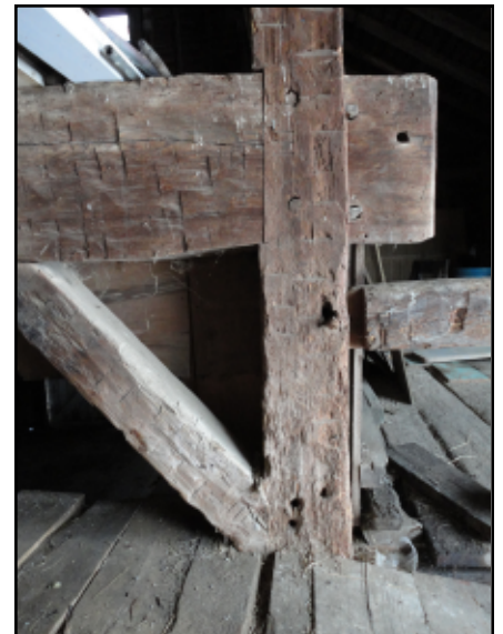
Photo 6. View looking north at the east end anchorbeam-post joint of bent 3 (January 2011).
