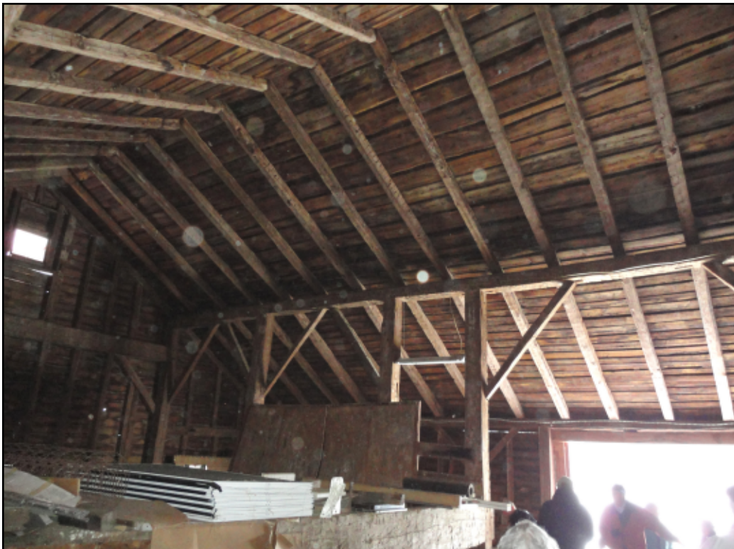
Photo 9. Interior looking northeast. The irregular spacing of the bents, resulting from the insertion of the wagon entry bay, can be seen in this image (January 2011).
