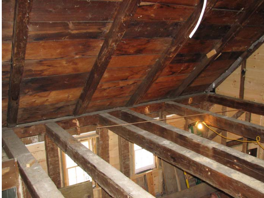
Figure 3. View in the attic of the Hills house, looking at the tops of six of the tying joints—from among 24 used in the main house and almost 30 more used in the two wings. In this one example, the use of “gunstock posts” was eschewed so that the posts could be concealed within plastered walls.
